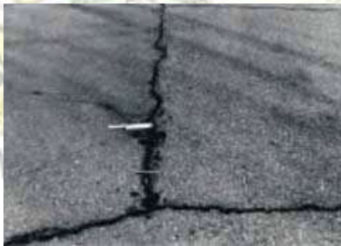
Gambar 2. 8 Retak Sambung ( Joint Refrection Cracking )
