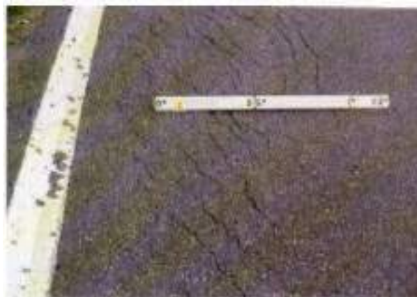
Gambar 2. 17 Patah Slip ( Slippage Cracking ) (Sumber: Bina Marga no.03/MN/B/1983)
