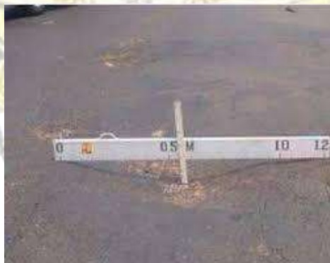
Gambar 2. 6 Amblas ( Depression ) (Sumber: Bina Marga no.03/MN/B/1983)
