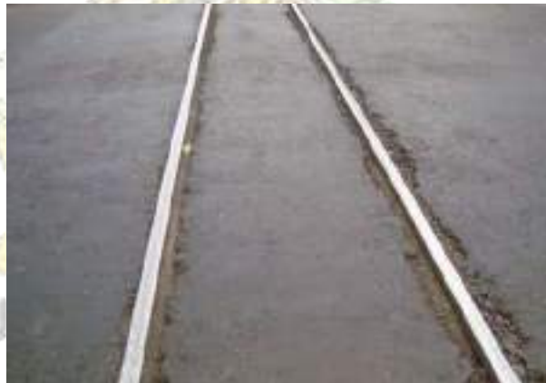
Gambar 2. 14 Rusak Perpotongan Rel ( Railroad Crossing ) (Sumber: Bina Marga no.03/MN/B/1983)
