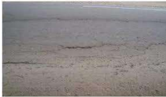
Gambar 2. 4 Cekungan ( Bump and Sags ) (Sumber: Bina Marga no.03/MN/B/1983)
