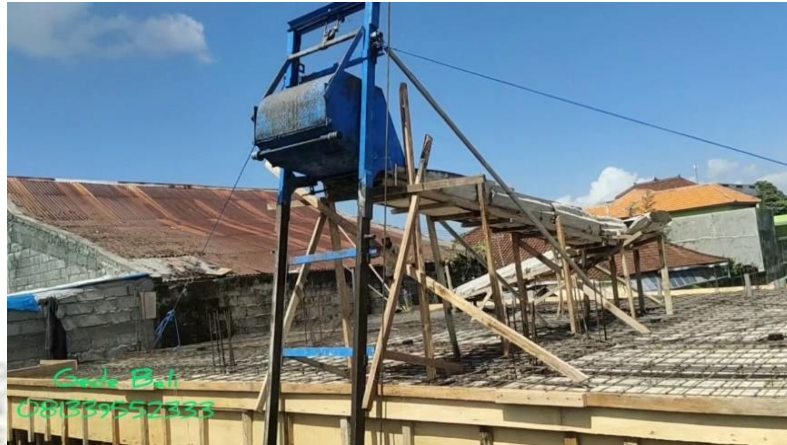
Gambar 22 Lift Cor (Sumber : Bali, G., 2020)
